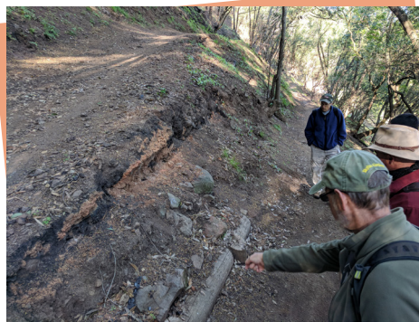
Joe Cavaness from V-O-Cal and Rick Fessenden from Skyline Park Citizens Association plan the repair of a destroyed retaining wall.
